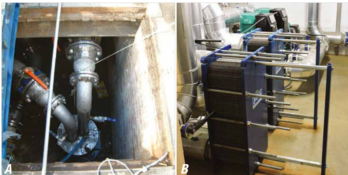
Fig 3: Two components of an open loop ground source heat system: (left) a water well - in this case installed with a submersible pump and reinjection main capable of abstracting/recharging up to 20 L/s (photo © David Birks) and (right) two plate heat exchangers (photo © David Banks).
